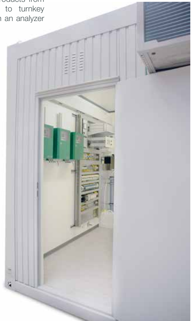
Analyzer house for emissions monitoring
